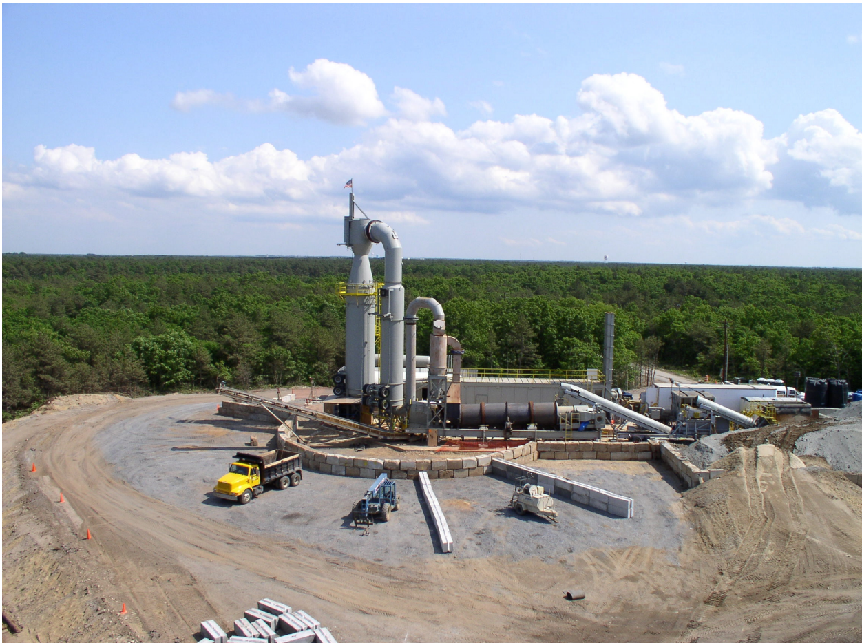
Mobile Thermal Treatment Unit
